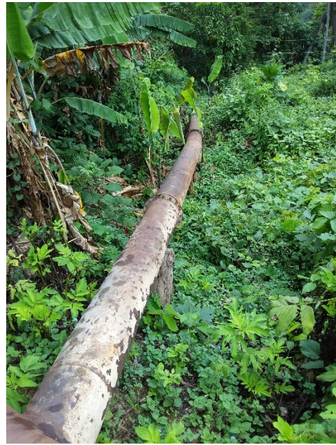
Figure 13 Water pipe of a mini-hydro powerplant
