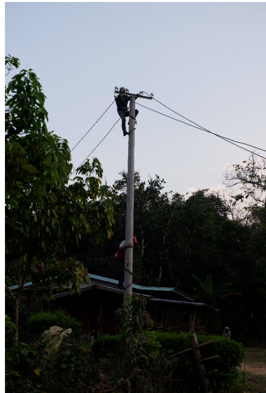
Figure 15 Wiring for a mini-grid
